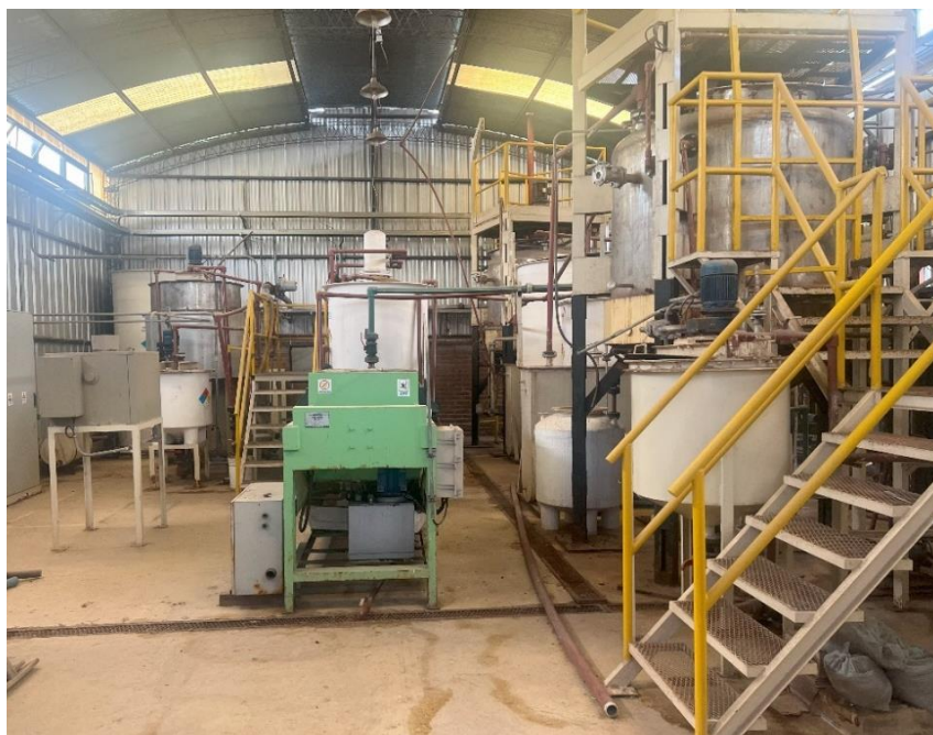
Pilot Plant during site visit March 2023. Source: Company
